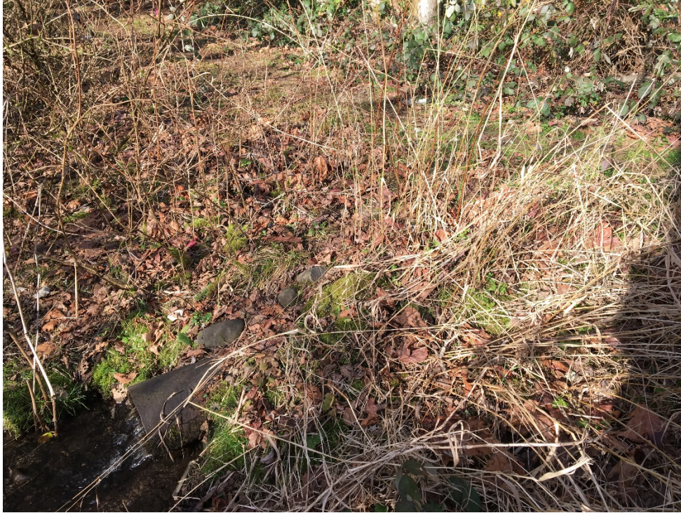
Photograph 7: Culvert outfall (bottom left) at the abandoned access road crossing where the boardwalk is proposed. Photograph taken January 14, 2018.
