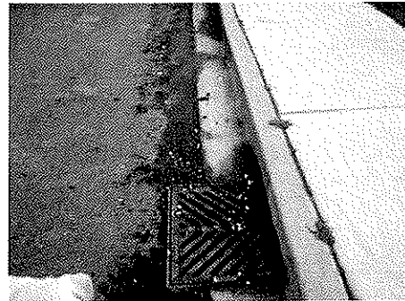
Latex paint residue on catch basin
